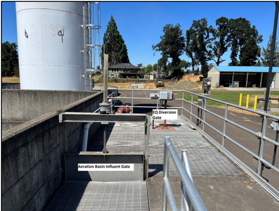
Figure 1. AB influent and EQ diversion gates
