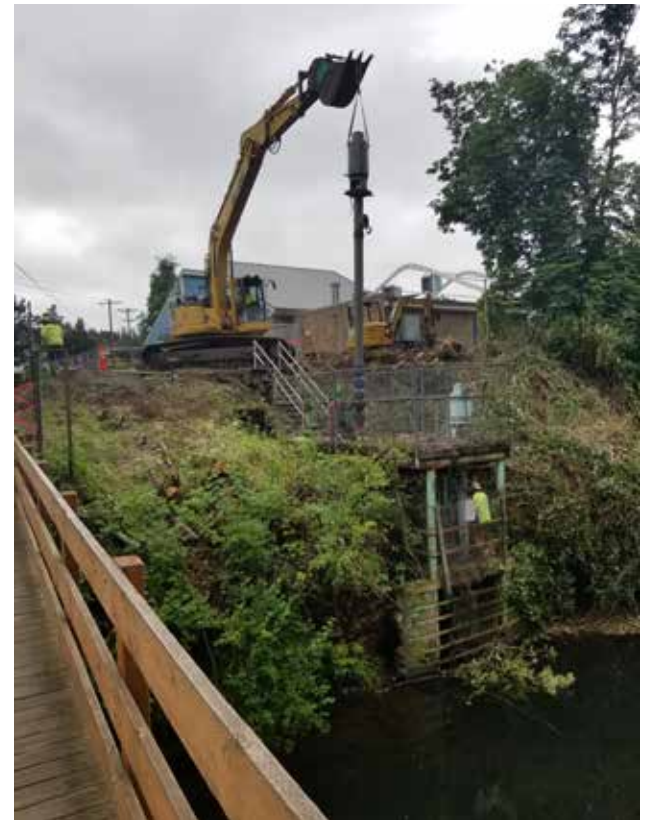
Crews have already been at work at the Silver Creek intake structure.
