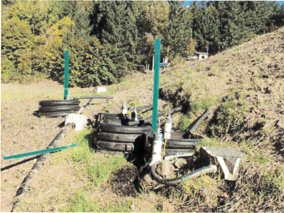
Toe drains and monitoring weirs
