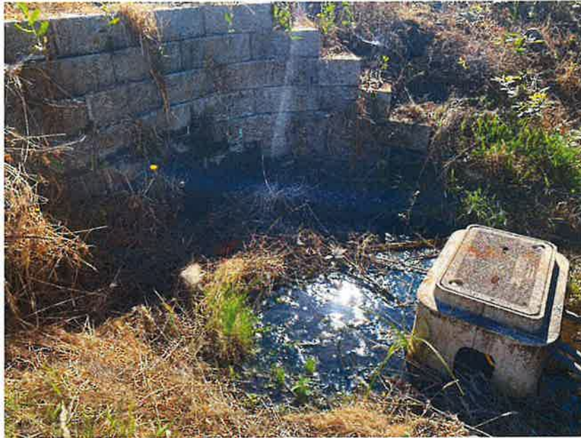
Typical seepage observed at reinforced area
