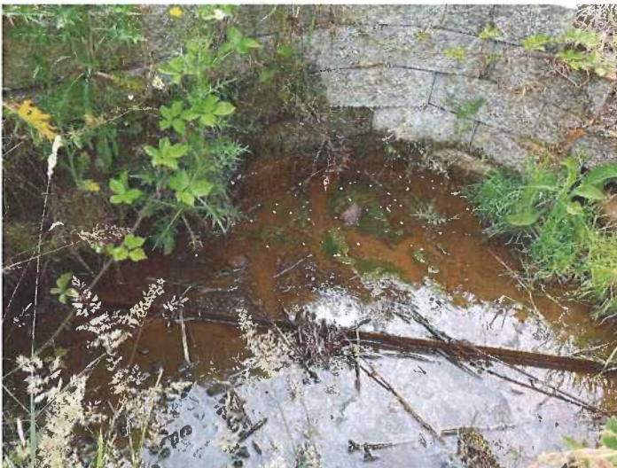
Area of seepage
