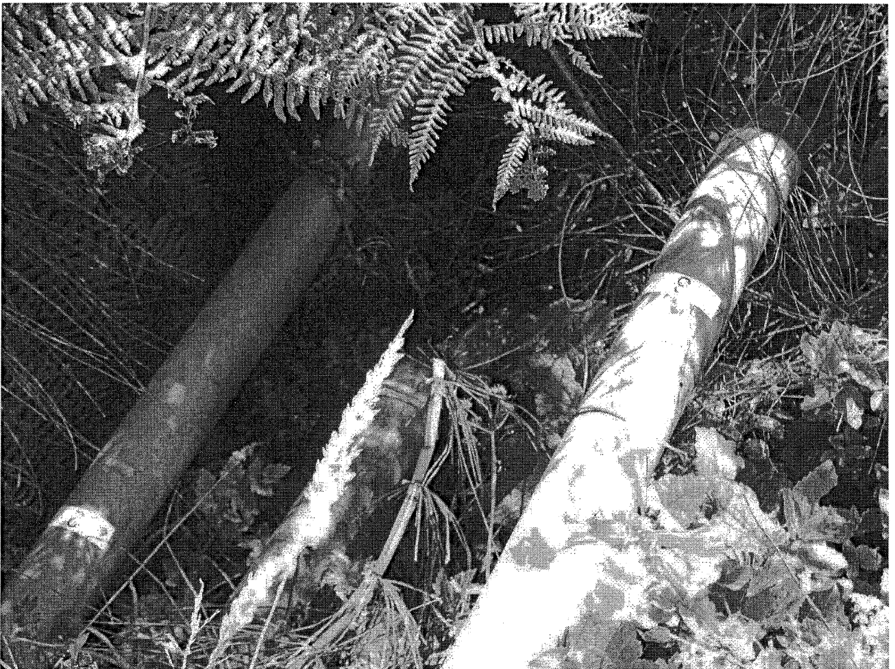
Figure 1a. Pipes 1,2,3 note that pipe 1 (middle) is flowing heavy while other two dripping.
