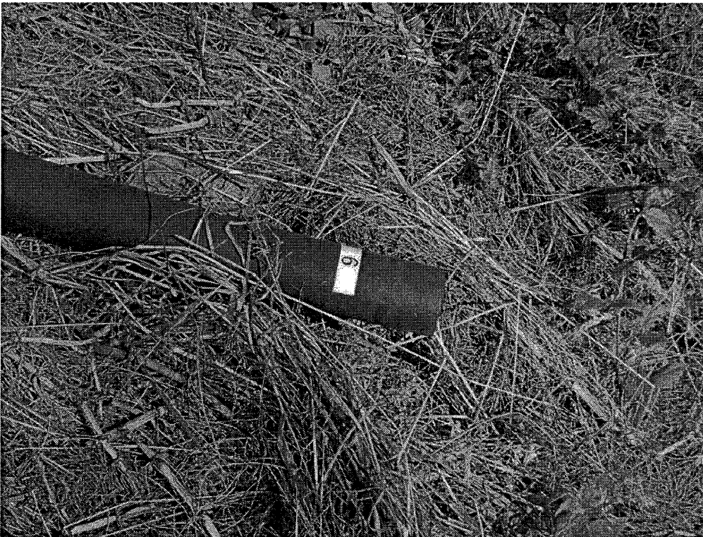
Figure 1e. Pipe 9 flowing lightly/dripping.
