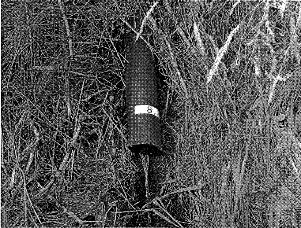
Figure d. Pipe 8 flowing lightly.
