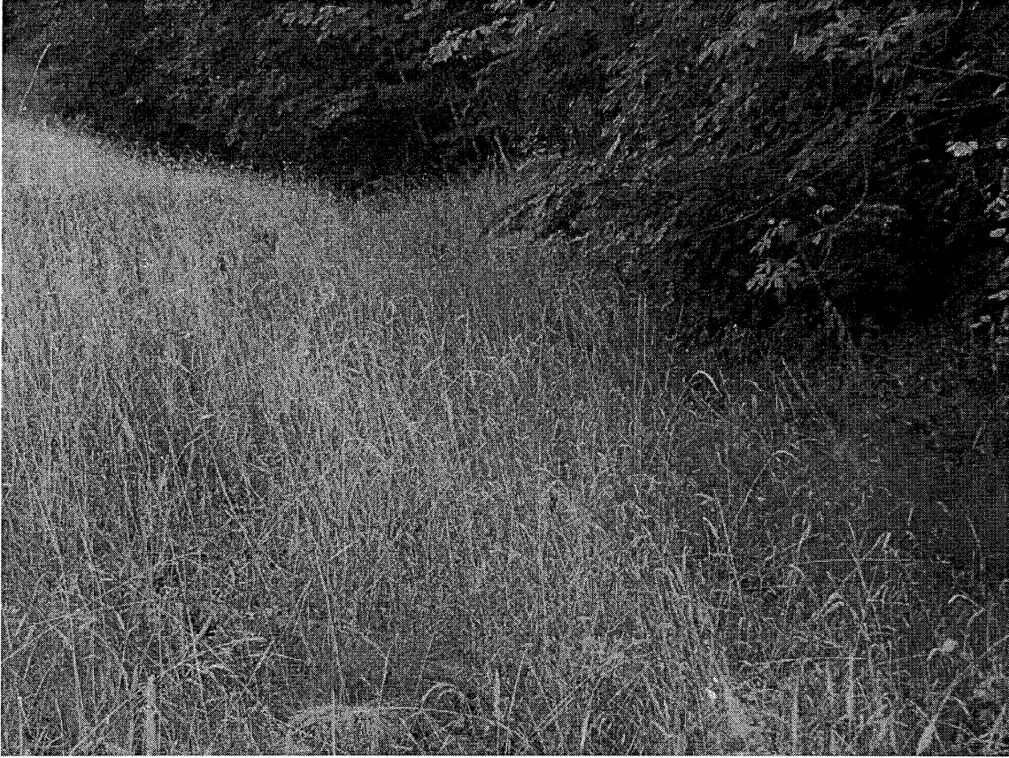
Figure 1f. “Seepage” or spring along left abutment with change in vegetation but no live water flowing.
