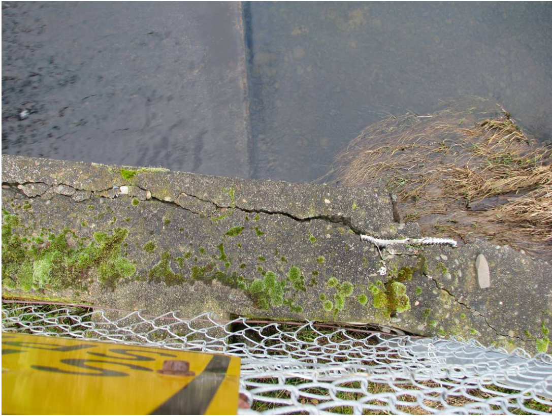
Figure 3. Spalling on dam spillway (left side facing downstream)
