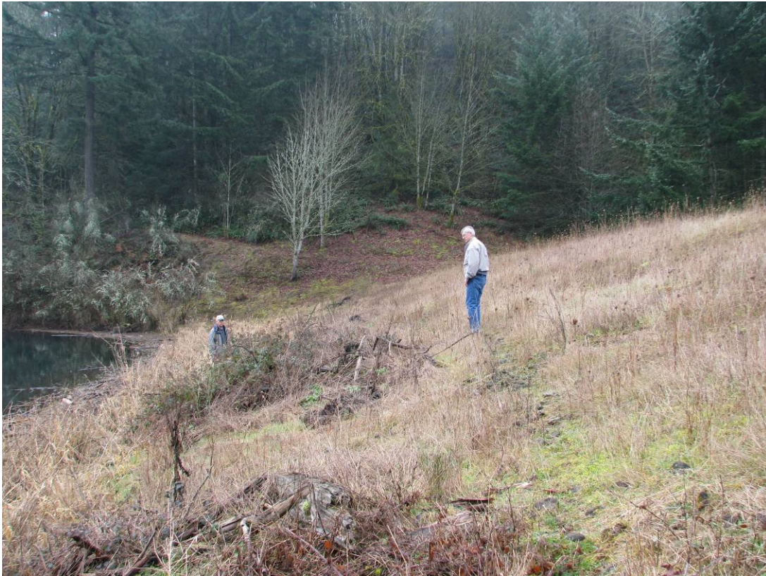
Figure 1. Vegetation on upstream face of dam.
