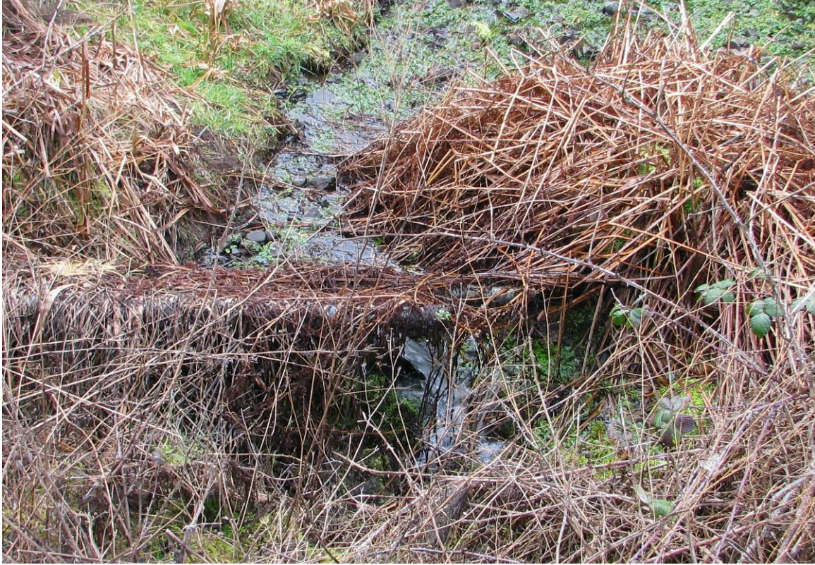
Figure 5. Seepage from toe drain (clear).
