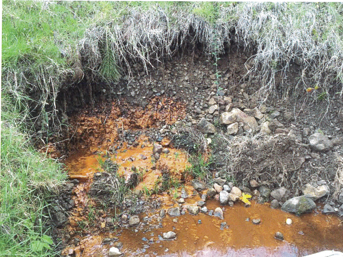
Excavated area of seepage above outlet
