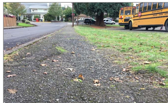
The north sidewalk on Robinson Street has deteriorated and is in poor condition.
