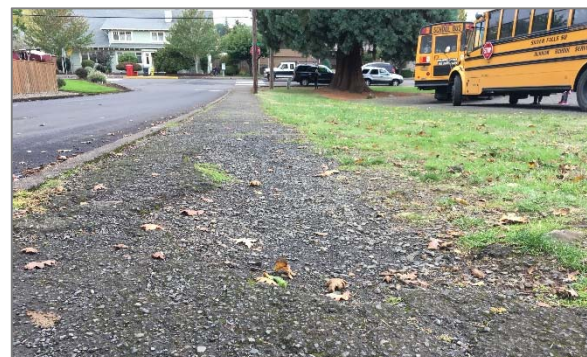
The north sidewalk on Robinson Street has deteriorated and is in poor condition.
