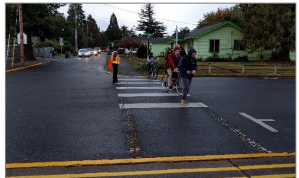
The main school crosswalk across Schlador Street and Brown Street lacks ADA-compliant curb ramps on both ends.
