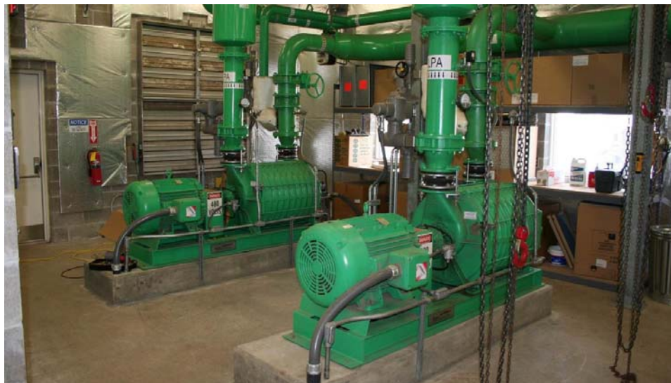
Figure 7-20: Silverton WWTP Blower Building
