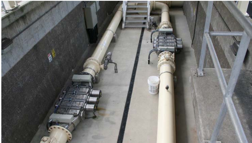
Figure 7-22: Silverton WWTP UV Disinfection System
