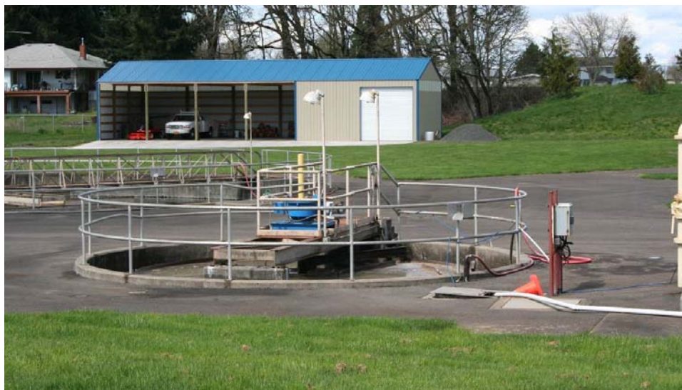
Figure 7-26: Silverton WWTP Primary Sludge Gravity Thickener
