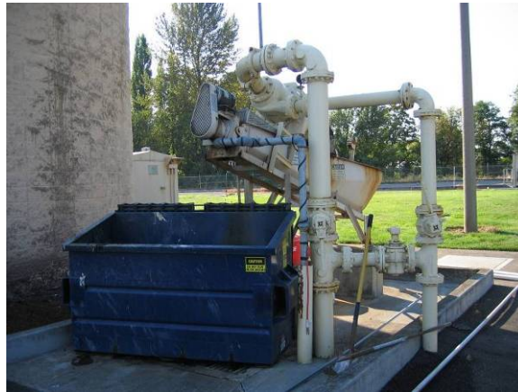
Figure 7-17: Primary Sludge Degritting Equipment
