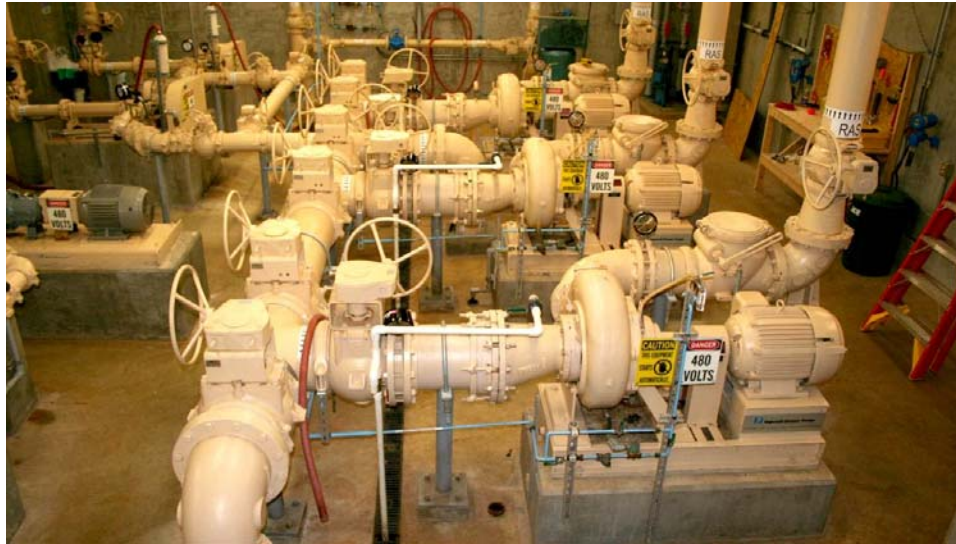
Figure 7-21: Silverton WWTP RAS/WAS Pump Station
