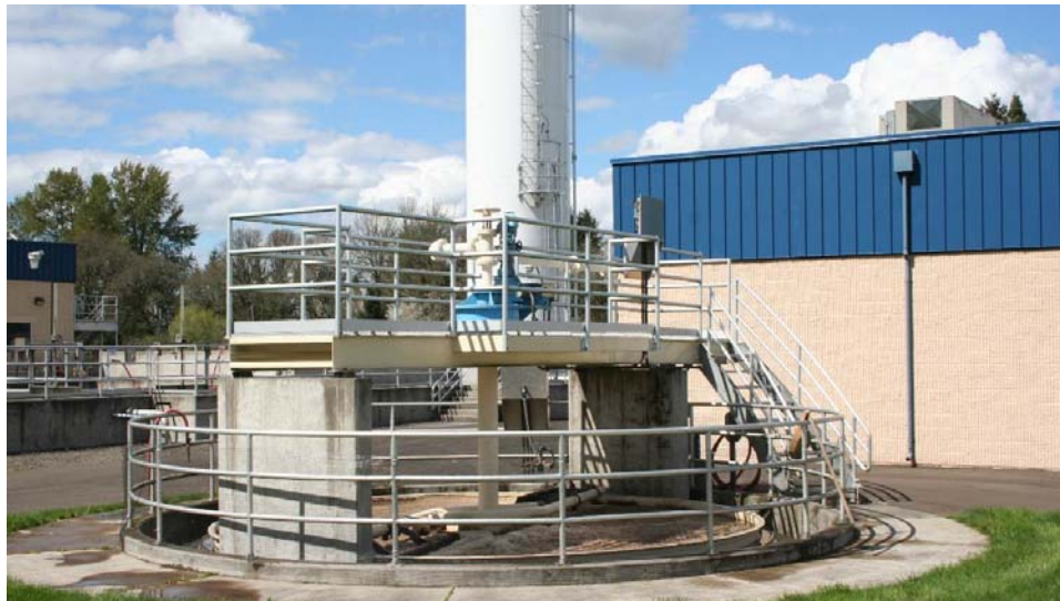
Figure 7-25: Silverton WWTP Dissolve Air Flotation Thickener
