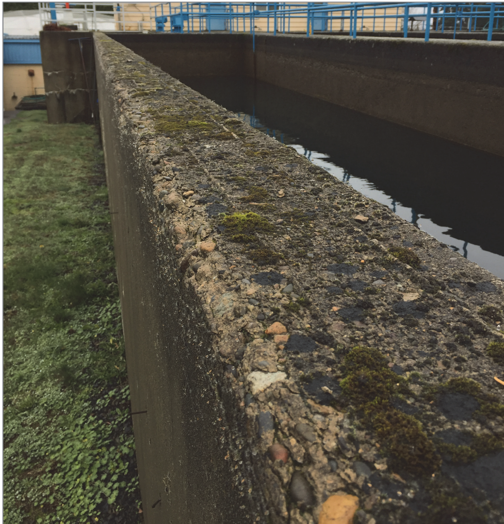
Exhibit 3.8 – Exposed Concrete Reinforcing
