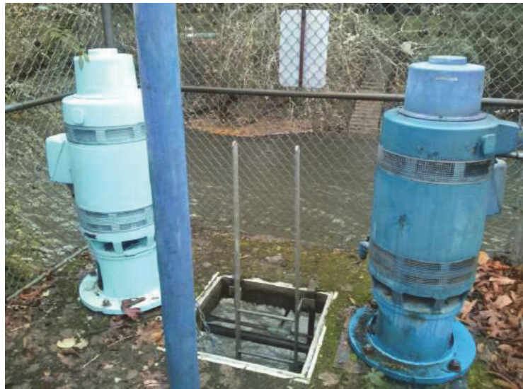
Exhibit 2.2 – Existing Silver Creek Pumps
