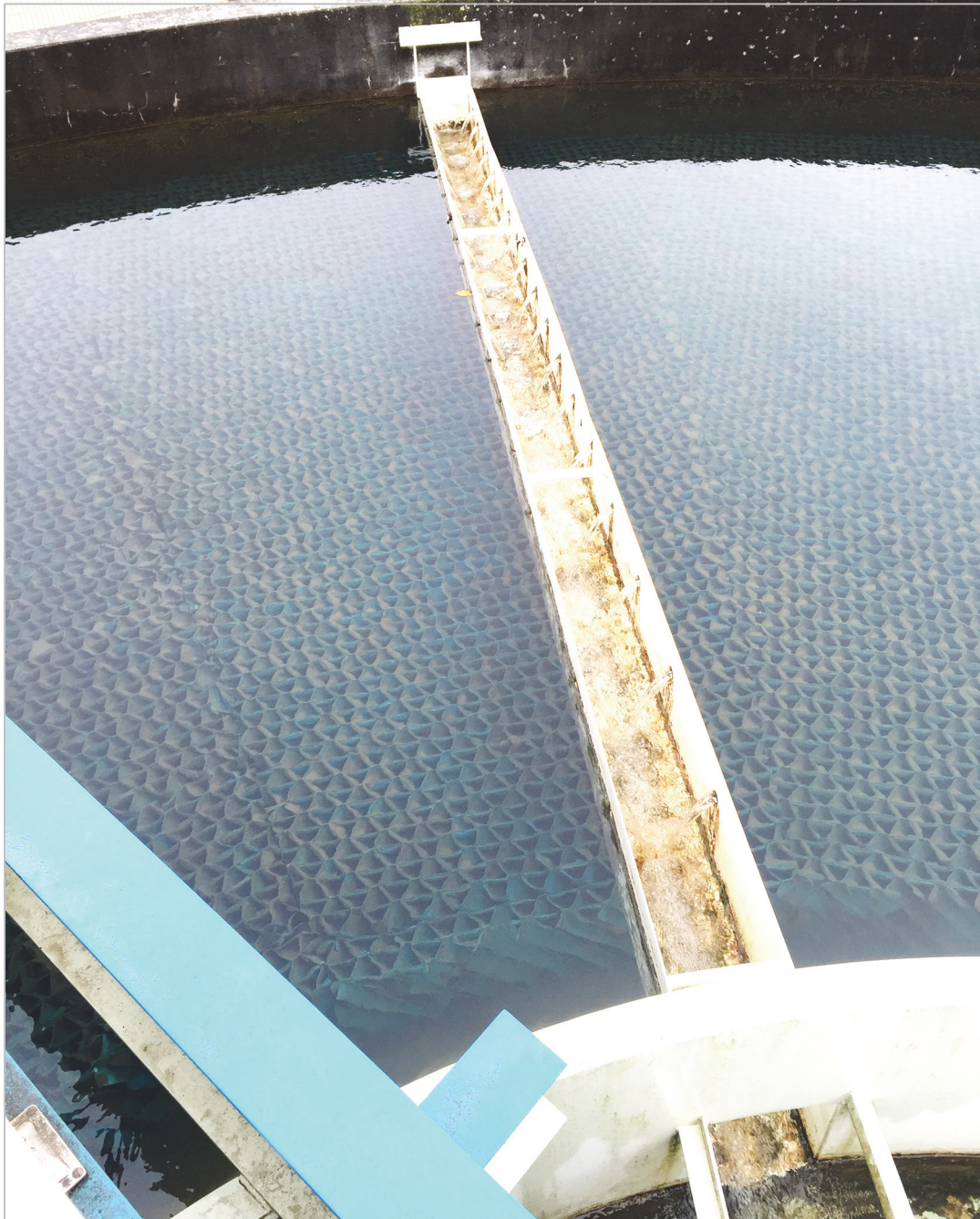
Exhibit 3.6 – Plant 2 Settling Tubes and Launder System (Silverton, Oregon)
