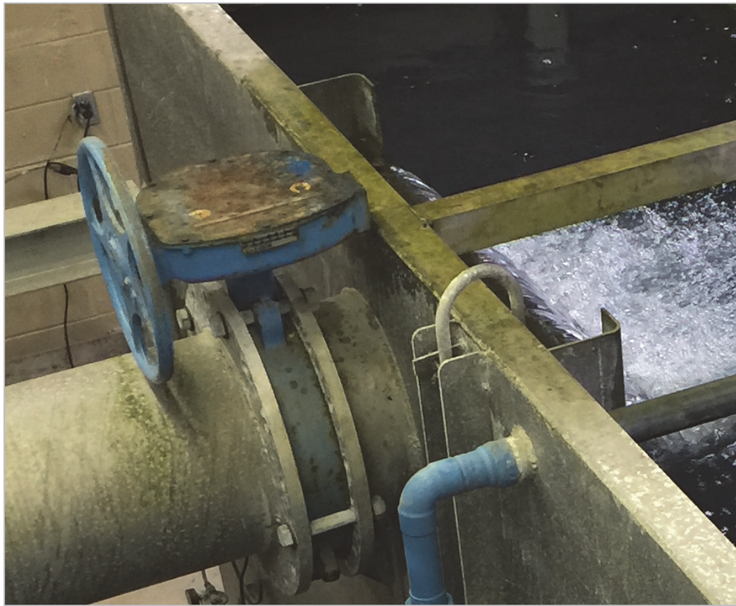
Exhibit 3.7 – Plant 2 Filter Inlet Line and Entrance Baffle
