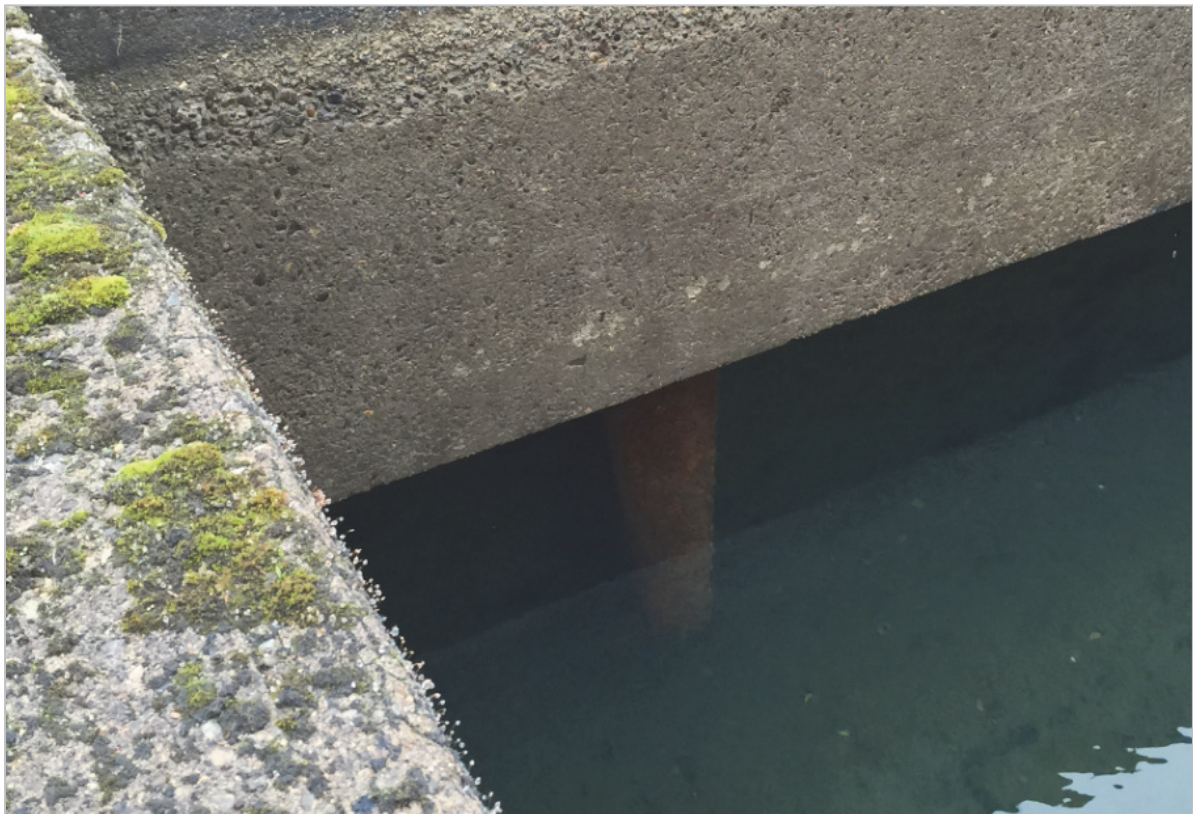
Exhibit 3.3 – Outlet Pipe Extending into Sedimentation Basin
