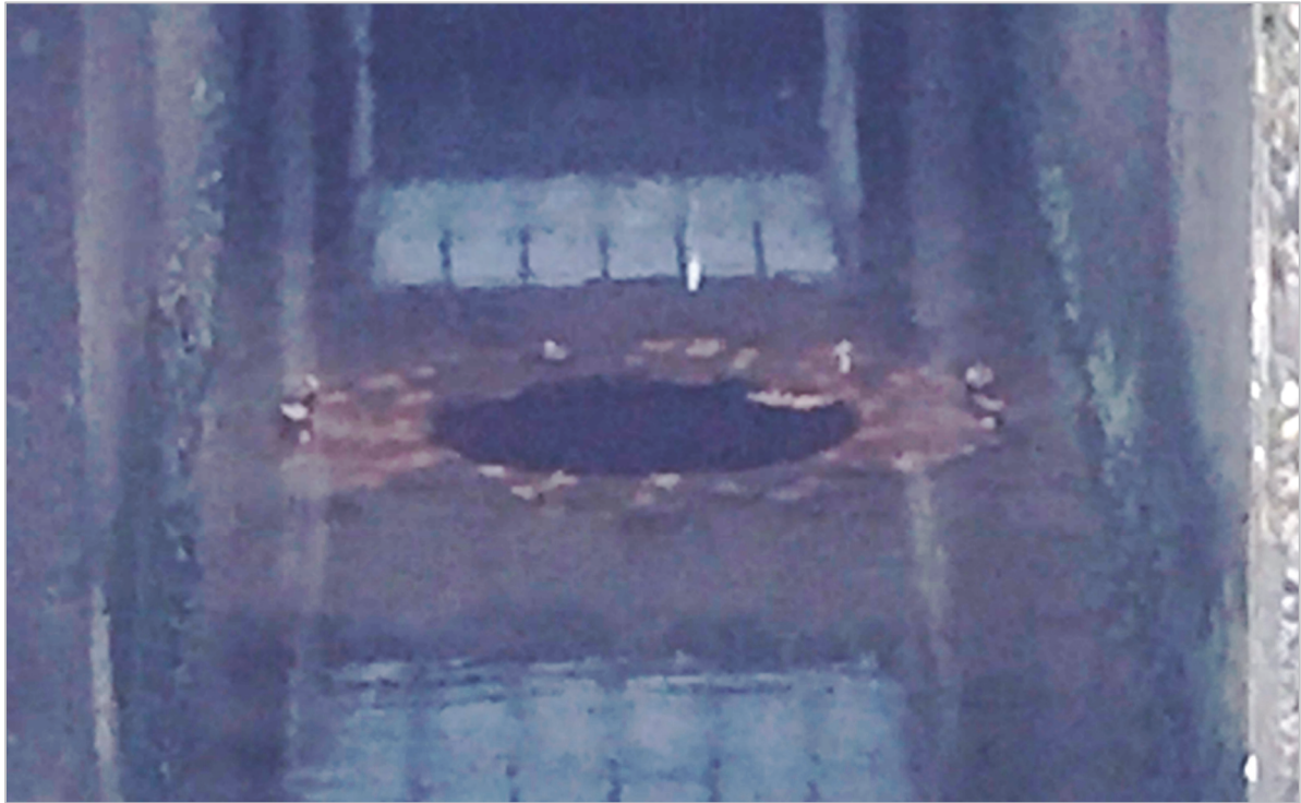
Exhibit 3.2 – Outlet Pipe Opening in Concrete Channel
