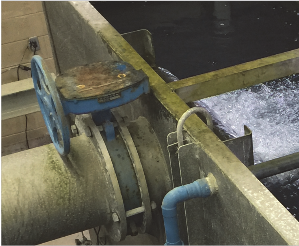
Exhibit 3.7 – Plant 2 Filter Inlet Line and Entrance Baffle
