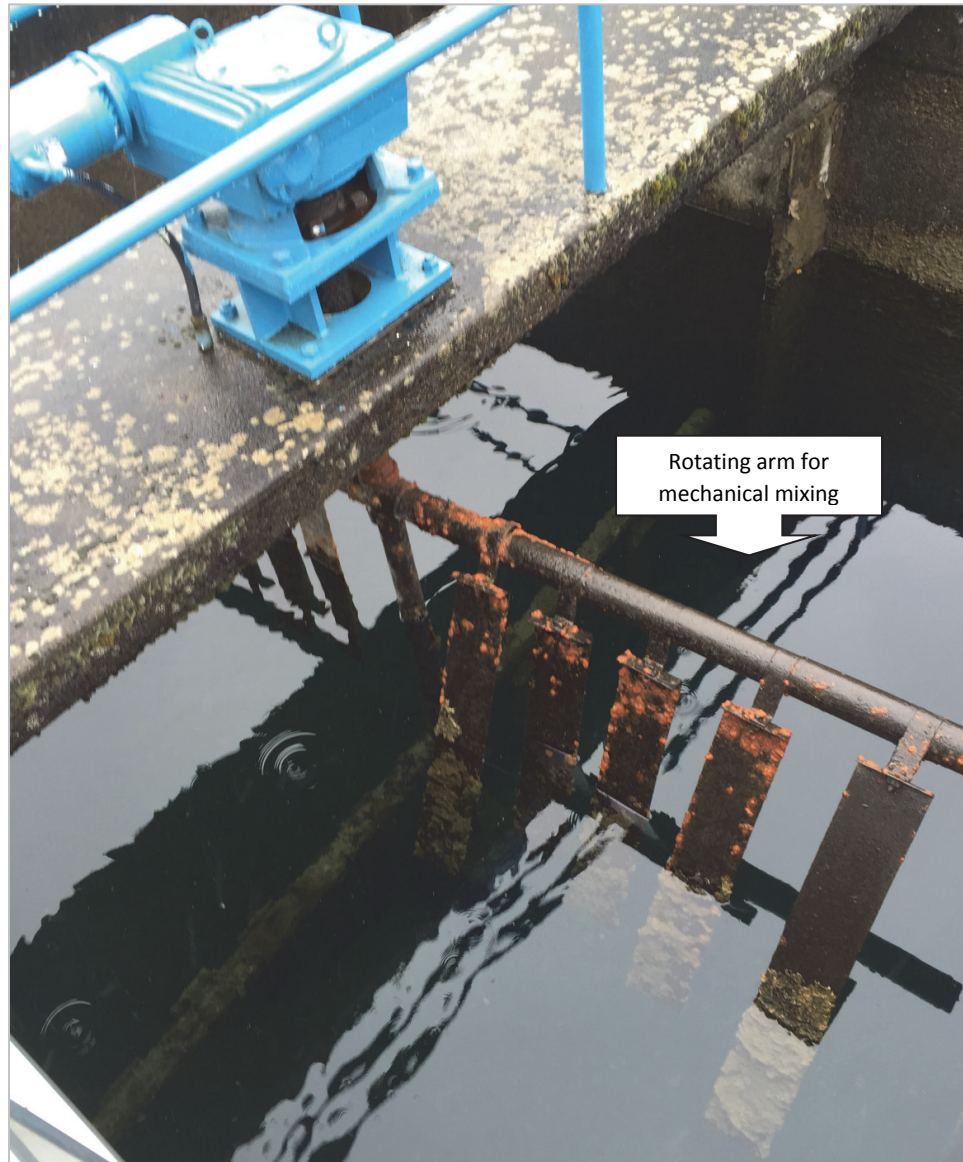
Exhibit 3.1 – Plant 1 Flocculation Basin 1
