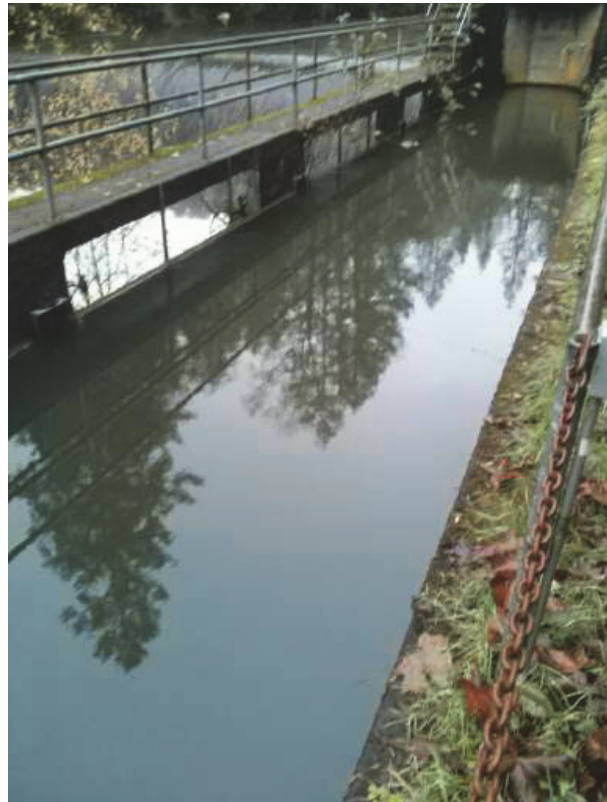
Exhibit 2.1 – Abiqua Sedimentation Basin
