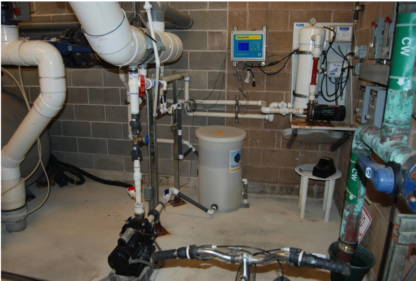
Location of Versa Chlor cal hypo feeder
