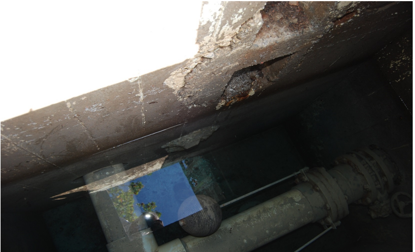
Image of original surge tank with wall degradation.
