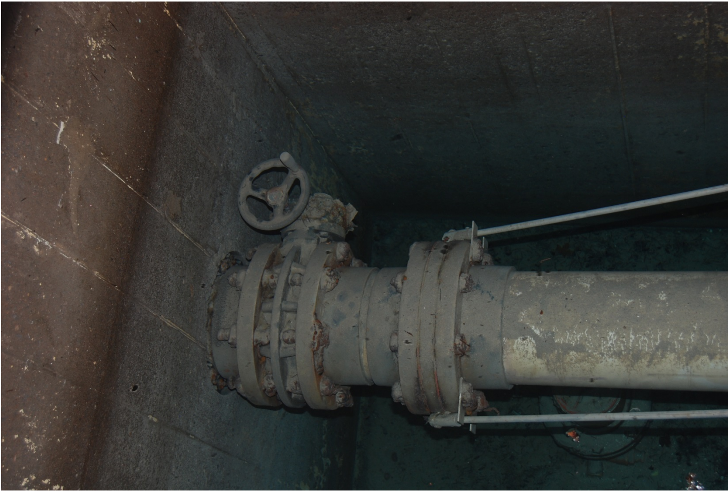
Image of original surge tank showing abandoned plumbing in floor and modulation valve.
