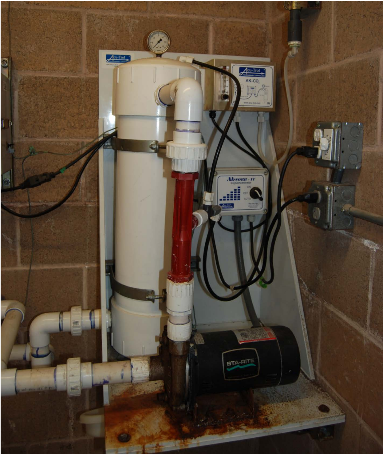
CO2 Venturi Feed System
