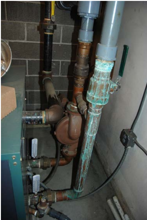
Mixed piping CPVC and Copper at Heater
