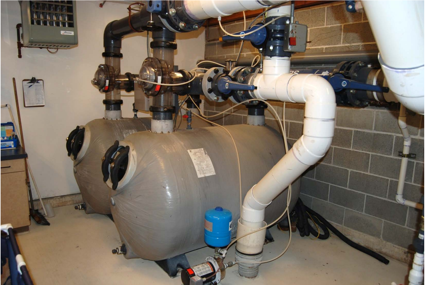
Example mixed PVC circulation piping material
