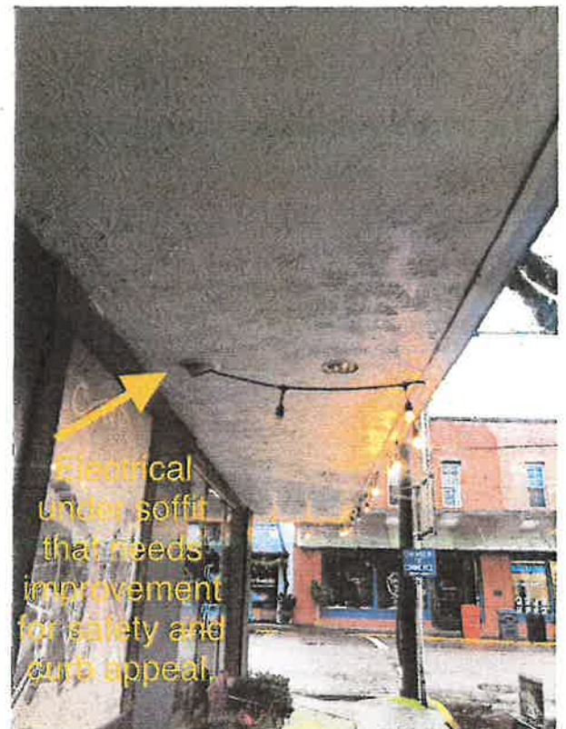
Figure 2B: Failing exterior lights under awning with string of lights coming out of fixture.
