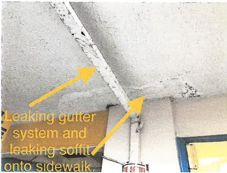
Figure 2A: Leaking gutters and leaking soffit that leak onto sidewalk.
