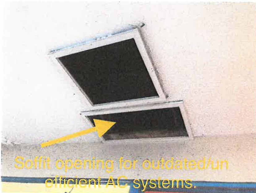
Figure 2C: Openings in soffits of awning that could allow pests to enter.
