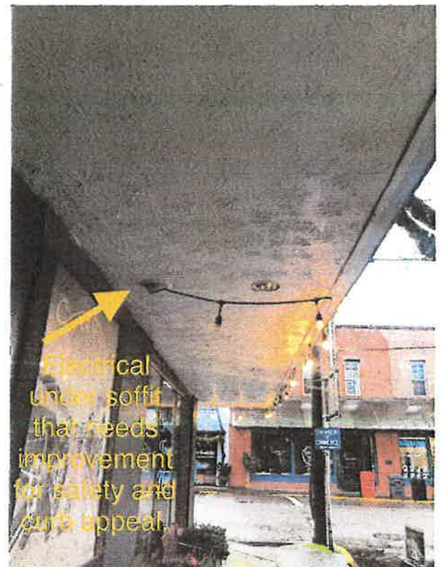
Figure 2B: Failing exterior lights under awning with string of lights coming out of fixture.
